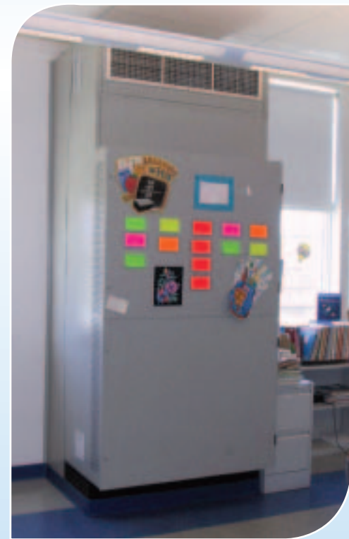
The Marvair Scholar II heat pump, which allowed the school system to keep construction costs under $14 per square foot, also serves as a showcase for student art.
